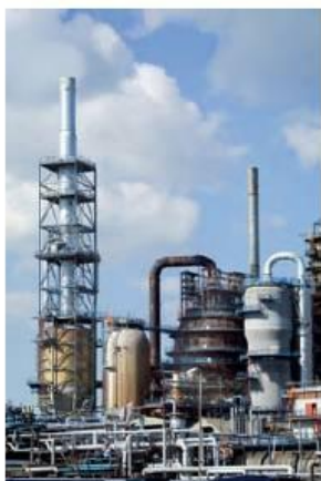
Figure 13.5 In a catalytic cracker (a 'cat cracker'), long-chain molecules are converted into shorter-chain molecules which have more uses.
