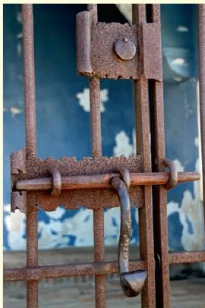
Figure 23.6 An untreated iron gate rusts when exposed to air and water.
