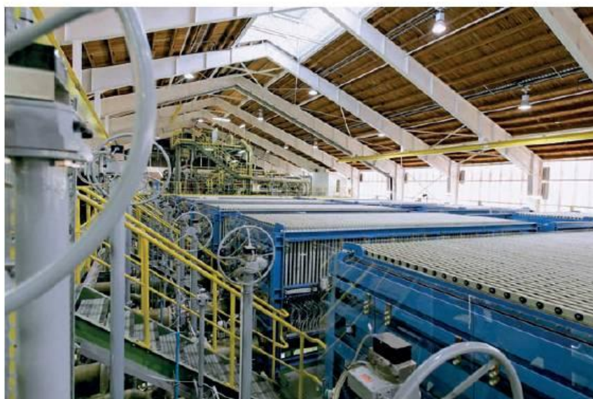
Figure 7.7 Modern plants use a membrane rather than a diaphragm in the cell. This yields very pure sodium hydroxide.
